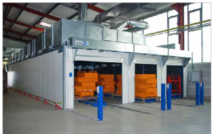
Paint shop with drying area
