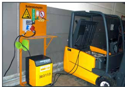
Battery Charging Station
