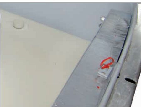
Dipstick to register any leakage
