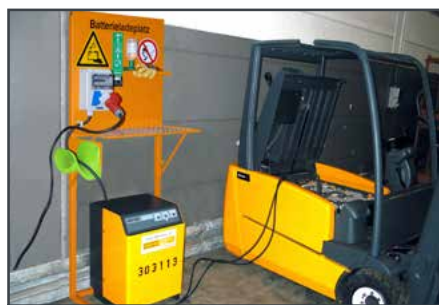
Station de charge de batteries
