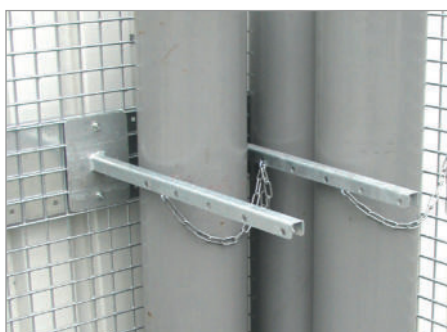
Fixture with safety chain
