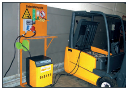
Battery charging station
