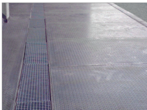
Drain channel with grate
