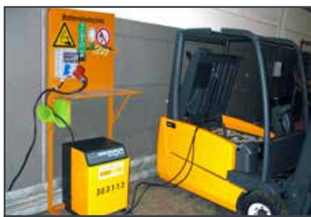
Station de charge de batteries
